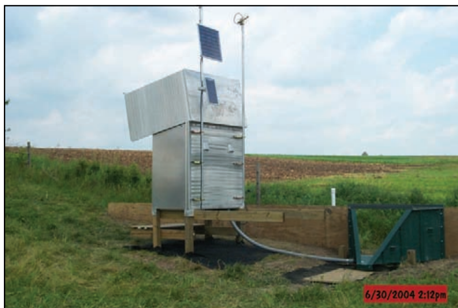
Figure 32: Solar powered edge-of-field site (H3)
