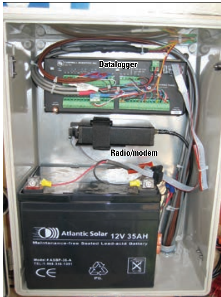
Figure 10. A Campbell Scientific, Inc., CR10X datalogger, an RF400 spread-spectrum radio/modem, and a battery were typically used for all edge-of-field, streamgaging, subsurface-tile, and meteorological stations.
