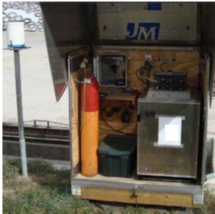
Figure 15: Sample equipment inside the enclosure.
