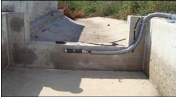
Figure 21: Sample & bubble line placement on the weir plate.
