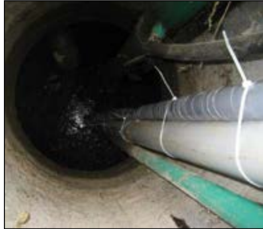
Figure 19: PVC pipe extending to tank bottom.
