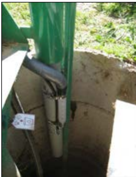
Figure 17: PVC pipe attachment.
