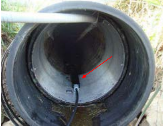
Figure 43: Area velocity flow meter installed.
