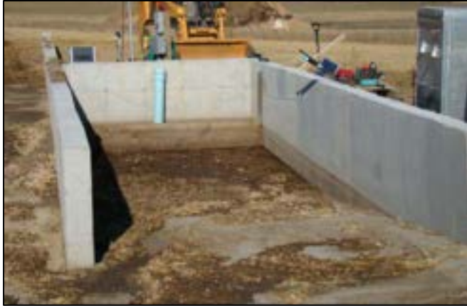
Figure 7: Retaining wall and collection sump (flotate trap).
