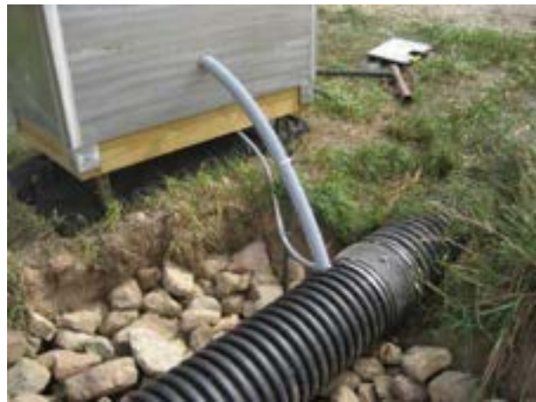
Figure 42: Sample and bubble line installed.
