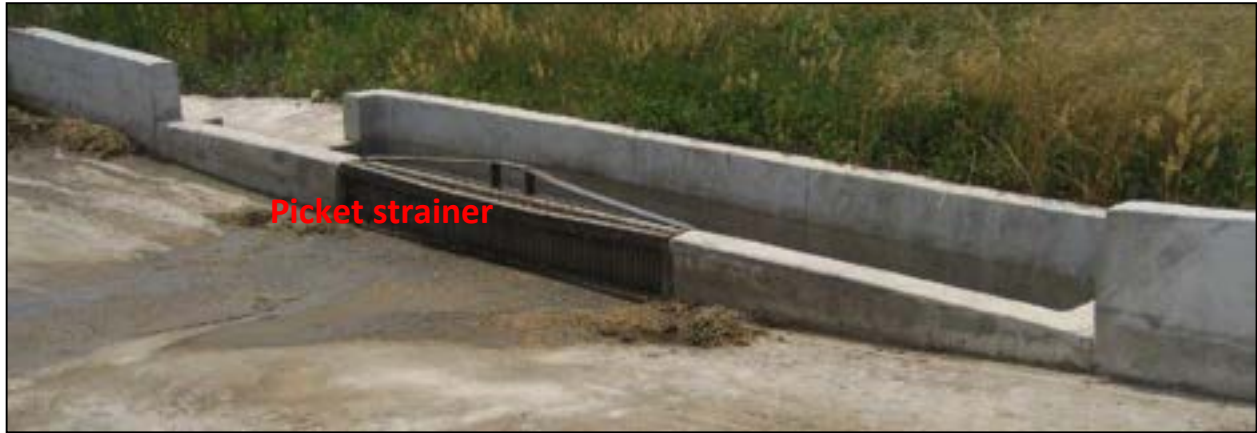
Figure 3: Particulate removed by picket strainer.
