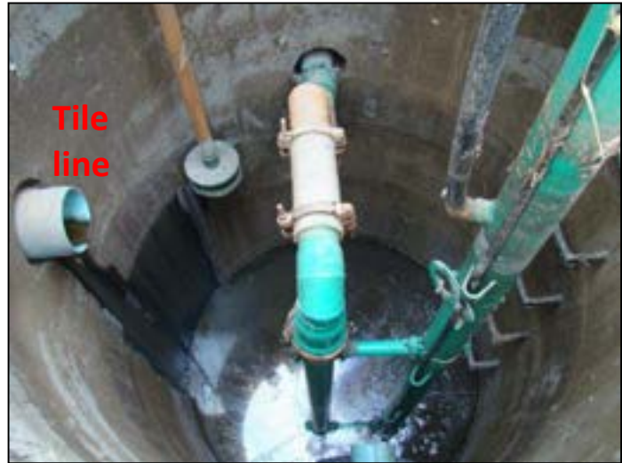
Figure 37: Tile drainage from bunker storage coming into the collection tank.
