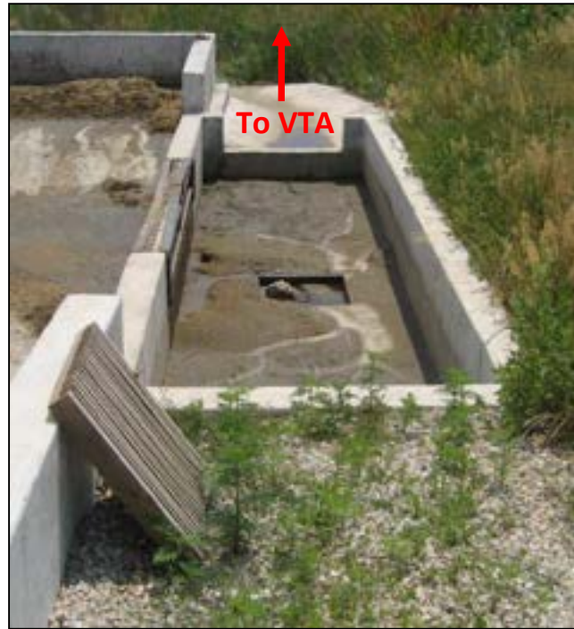
Figure 5: Sump overflow to VTA.
