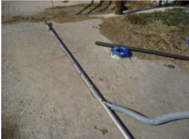
Figure 39: Lines attached to stainless steel pipe.
