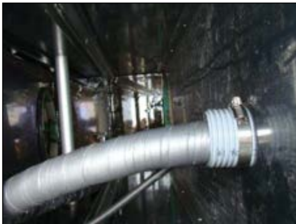
Figure 35: Sample and bubble line in Agri Drain.
