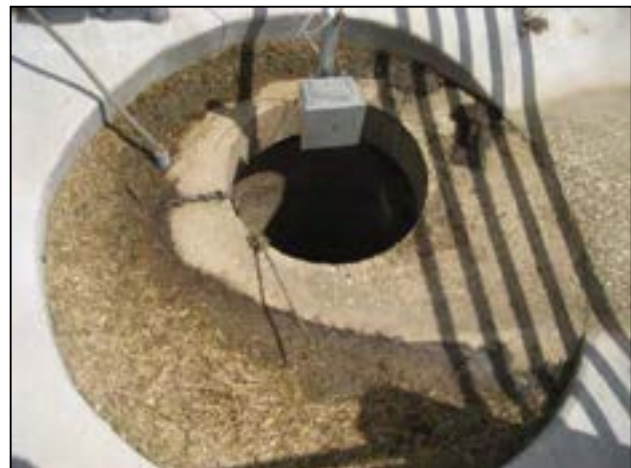
Figure 11. Liquid flows into manhole at the top of the collection tank
